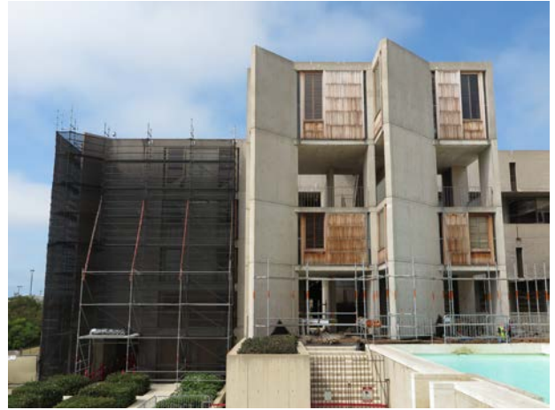
Construction activities underway at the west office wing (left) and study towers (right), summer 2016 Photo: J. Paul Getty Trust
